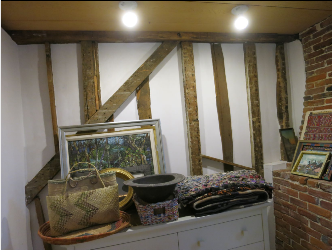
Second floor, studs and bracing for wall between front room and lean-to, Chimney on right.
