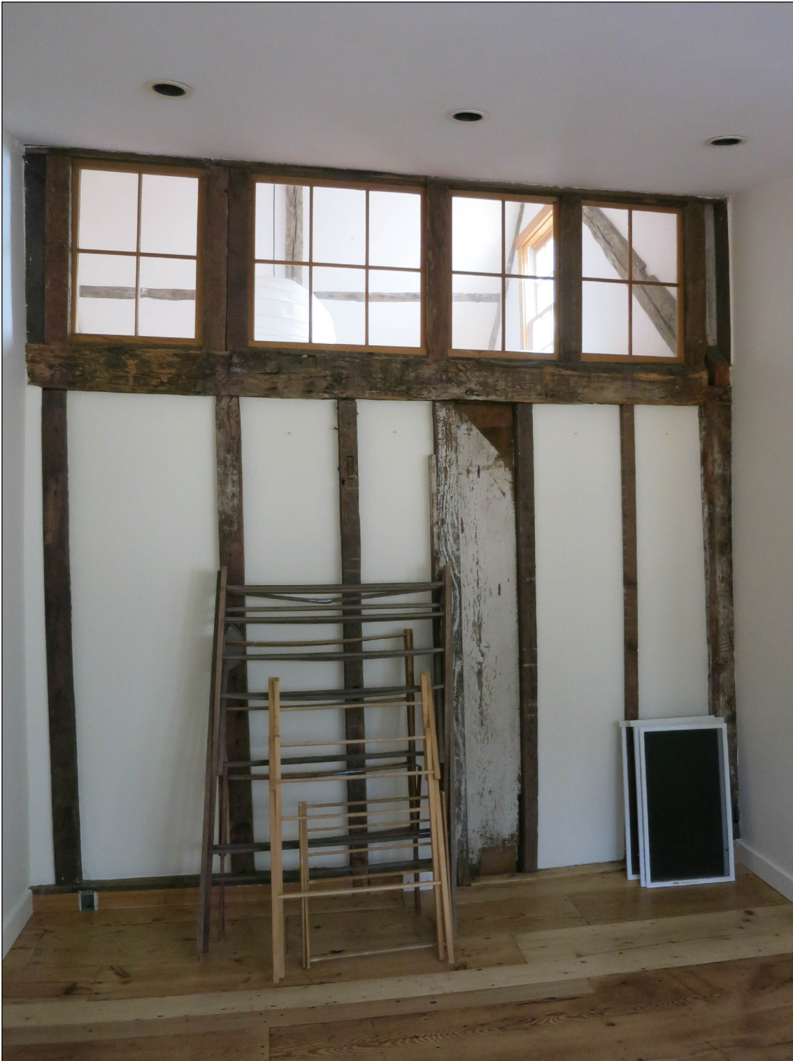
Second floor, lean-to, interior partition showing framing. Original roof followed rafter in end wall of front room (upper right) to beam below windows. The pitch was later raised to a plate above the windows and a shed dormer raised the roof even more.
