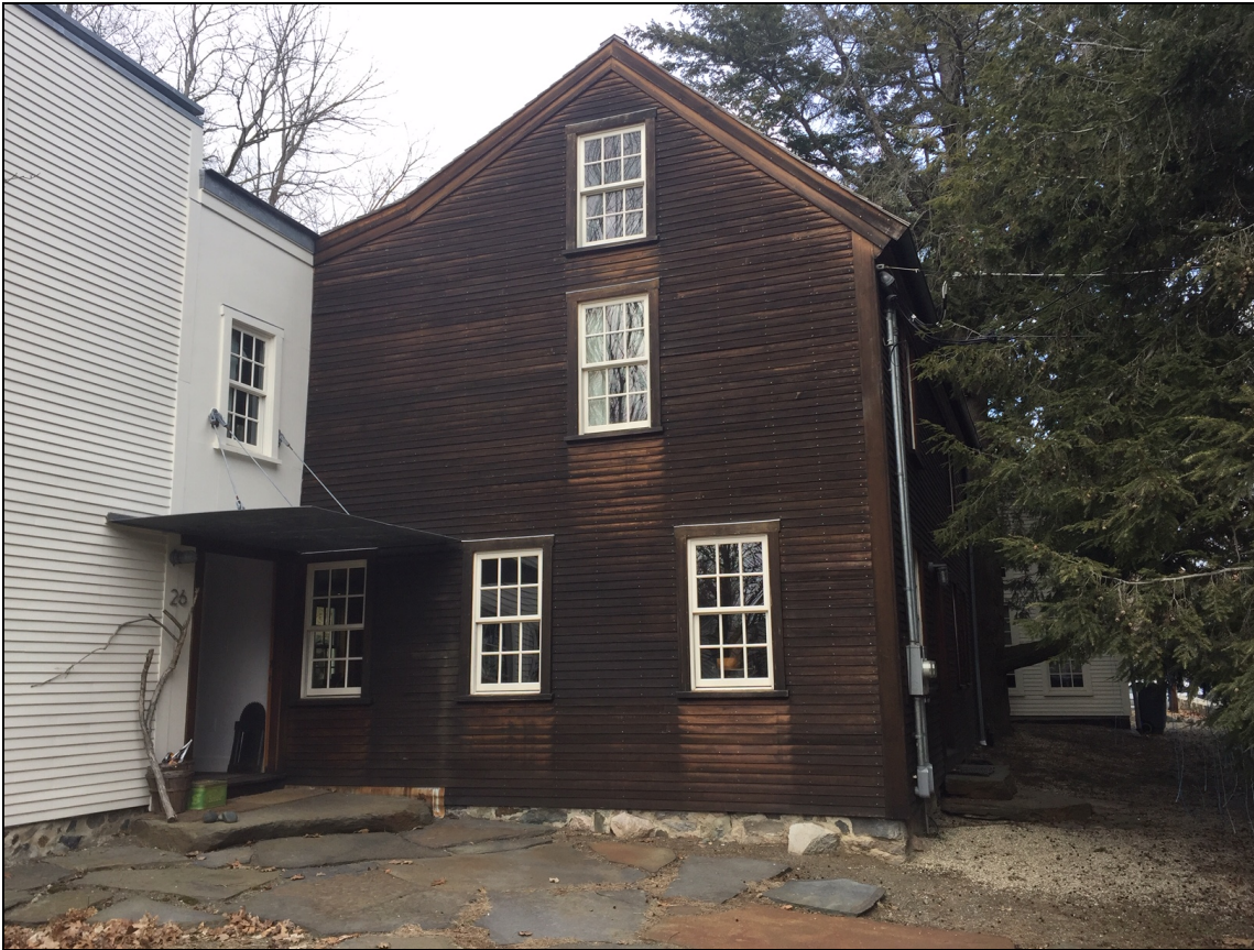
View of south end of house. Hyphen at left has a timber frame.
