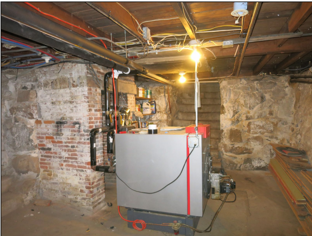
Basement looking north. Chimney base on left and north stairs in background.
